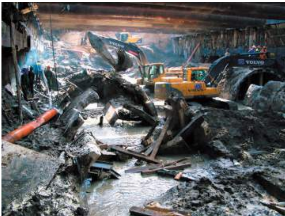
Fig 3.10.3. The consequences of a quicksand breakthrough in a subway tunnel under construction, Moscow, Russia http://biryulevo.ru/_fr/46/8590220.jpg
