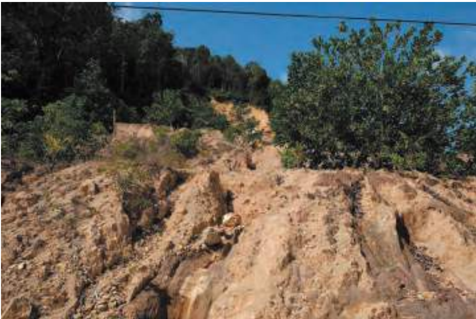
Fig. 3.7.1. Slope destruction by water erosion, Thailand. Photo by V. Benko
