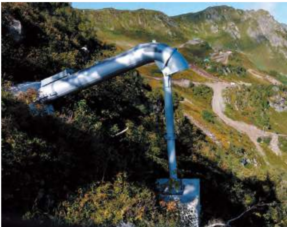
Fig. 3.5.17. The main part of the GazexExploder system is the installation of an active impact. It is a system of metal pipes for supplying the gas mixture directly to the collection, to which the gas pipes from the tanks located in the command post are connected. Inside the explorer, oxygen and propane gases are mixed in the ratio of 1 : 6
