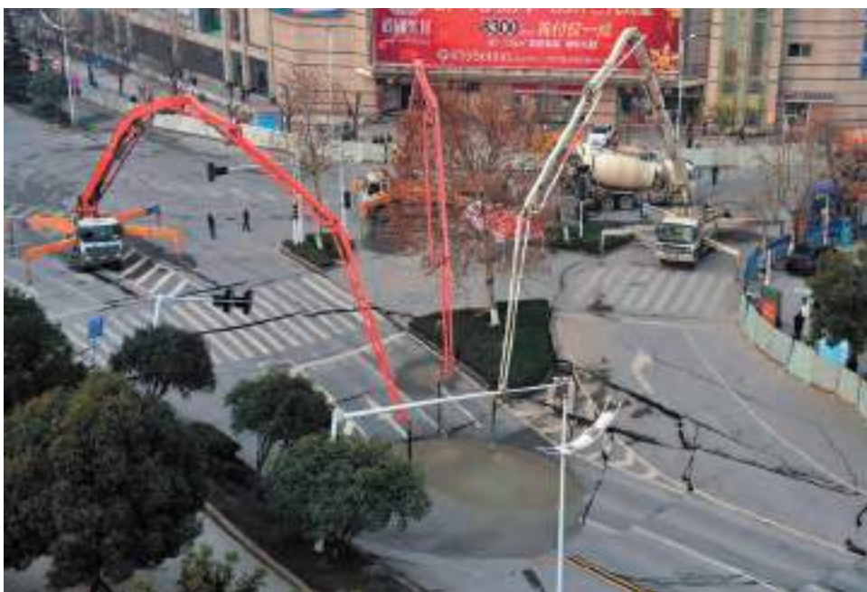
Fig. 3.11.6. Remediation of failure that occurred during the construction of a subway using concrete filling in Wuhan, China http://cs7054.vk.me/c7005/v7005554/2499b/TSSVvDmqhPg.jpg
