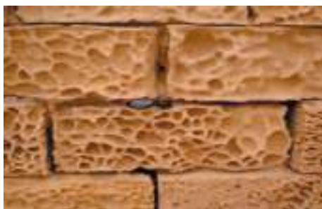
Fig. 3.6.9. Masonry Corrosion, Gozo Island, Malta
