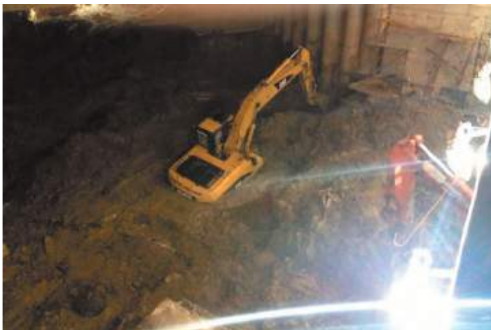
Fig. 3.10.11. Breakthrough of quicksand in an excavation in Kiev http://kievnews.glavcom.ua/media/o-00006717-n-00014261.jpg
