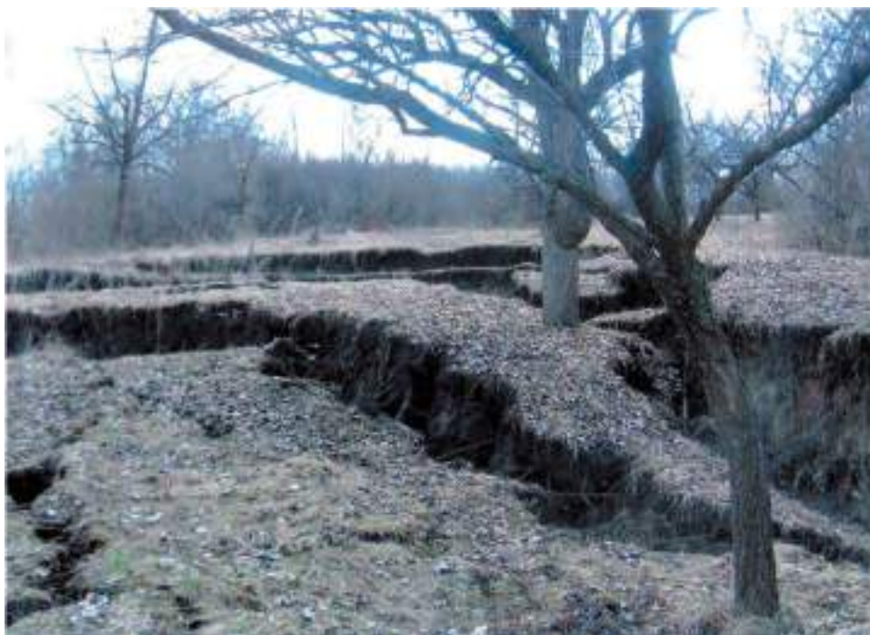
Fig. 3.4.4. Typical cracks on the upper part of the landslide slope Photo by G. Strizhelchik
