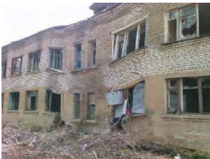
Fig 4.5.9. Destruction of the school building as a result of subsidence of the loess layer in the middle of the building https://engiserg.files.wordpress.com/2015/10/92-2.jpg? W = 648
