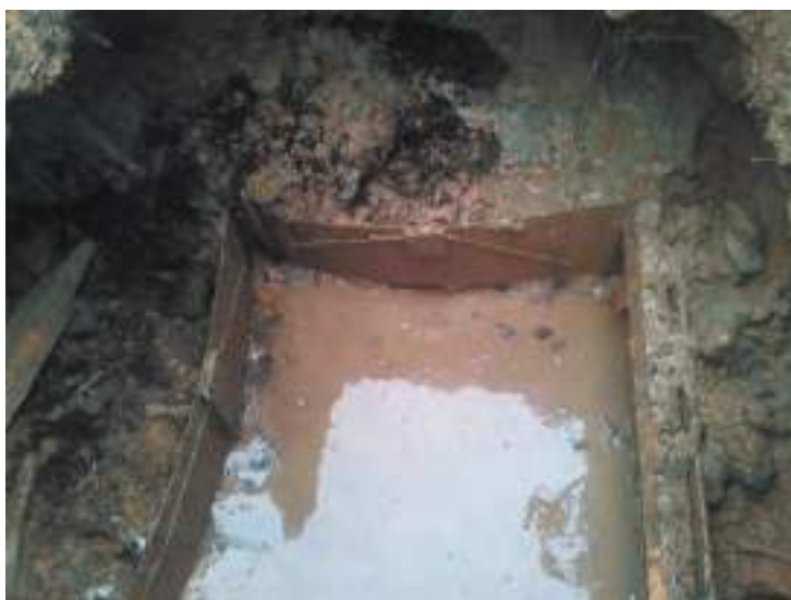
Fig. 3.10.1. Quicksand in the construction pit http://s001.radikal.ru/i193/1304/9f/5e40a1f7f302.jpg
