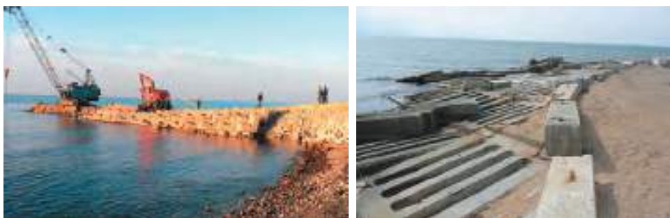
Fig 3.9.15. The use of reinforced concrete elements of various shapes for protection against abrasion http://ecodevice.com.ru/photogallery
