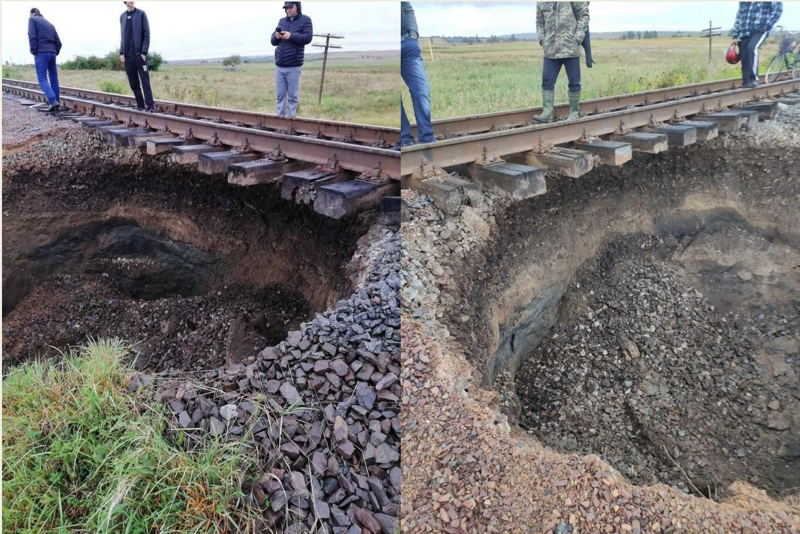
Fig. 20 Karst failure in Bukovyna. September 2021
