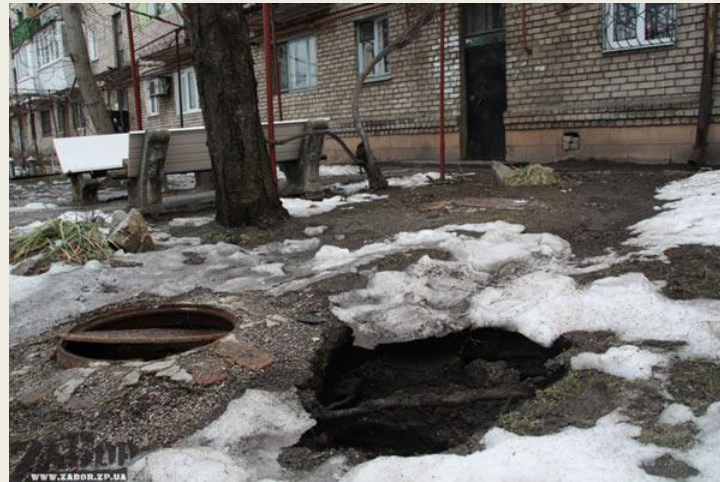
Fig. 4 Deformation of the pavement surface caused by suffusion and movement of soil into the manhole
