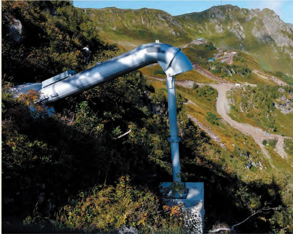
Fig. 46. The main part of the Gazex Exploder system is the installation of an active impact. It is a system of metal pipes for supplying the gas mixture directly to the collection, to which the gas pipes from the tanks located in the command post are connected. Inside the explorer, oxygen and propane gases are mixed in the ratio of 1 : 6
