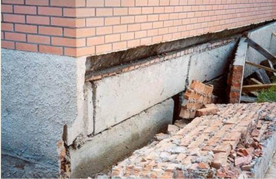
Destruction of the foundation during the subsidence of the underlying loess strata
